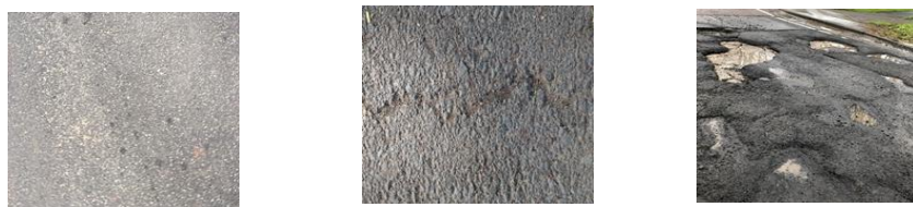
a. Road image not damaged b. Cracked Road c. Cracked potholed road
