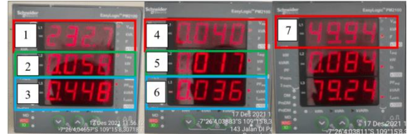
Fig. 23 Electrical value on Display Power Meter (End to End Measurement)
