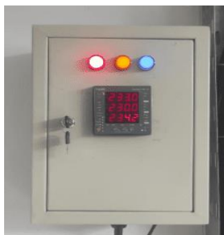
Fig. 16. Power Meter Panel Installation Results
